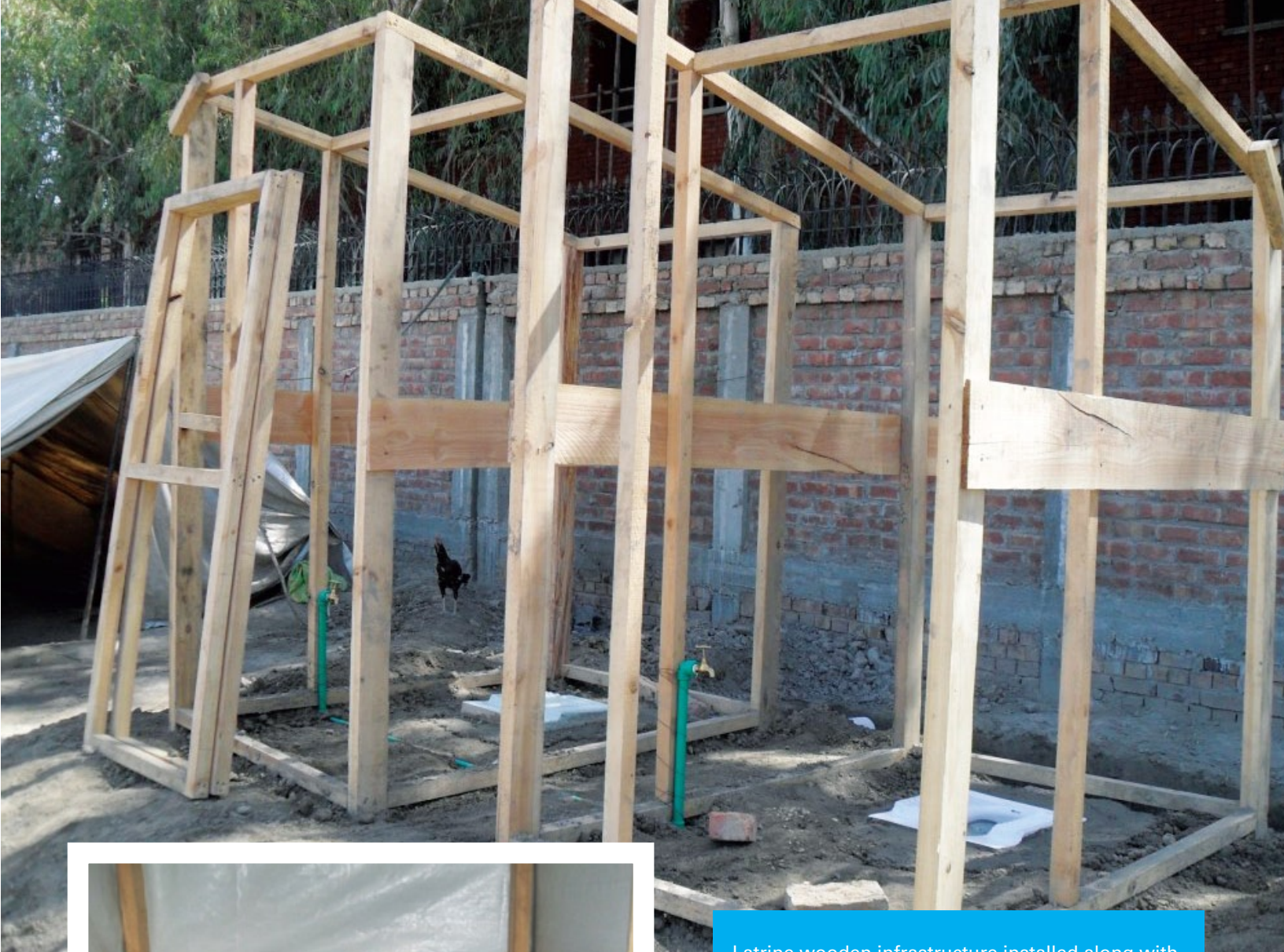
Latrine wooden infrastructure installed along with pour flush pans (above) and completed latrine with plastic sheeting walls (left)
