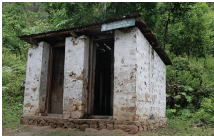
Poorly maintained school pit latrines.
