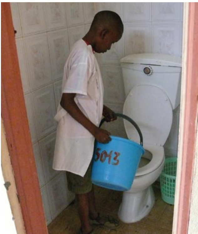
Flushing a toilet with a bucket of water at a primary school in Luanda.
