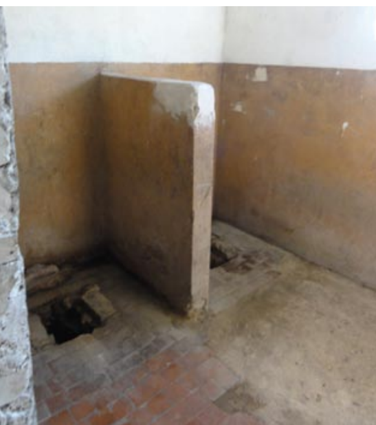
Inadequate pit at a public school in the village of Atskuri, Akhaltsikhe District.
