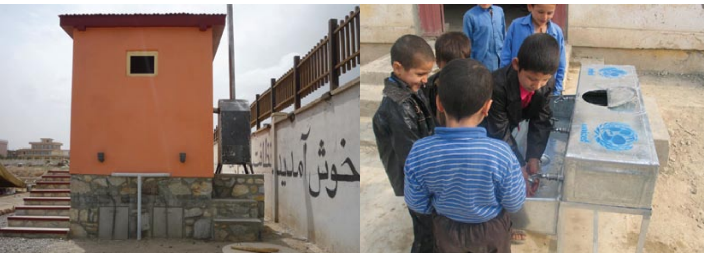
Eco-sanitation latrine at Wahdat girls' school, Kabul ( left ) and hand-washing facility at Raies Abdulkhalq school in Mazar City.
