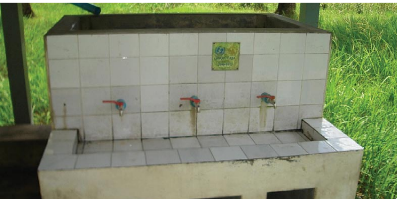
Hand-washing facility at a primary school in Pyapon District, Myanmar.
