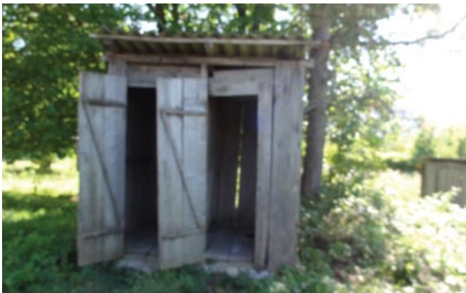
Rundown latrine at a public school in the village of Lasuriashi, Tsageri District.
