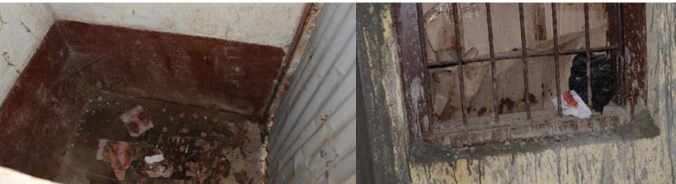
Dirty, unused toilet in a Kathmandu School (left) and no disposal system for used sanitary pads.
